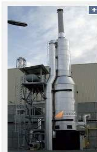
A vertical thermal oil heater at Kronospan, Sebes, with air pre-heater and stack
